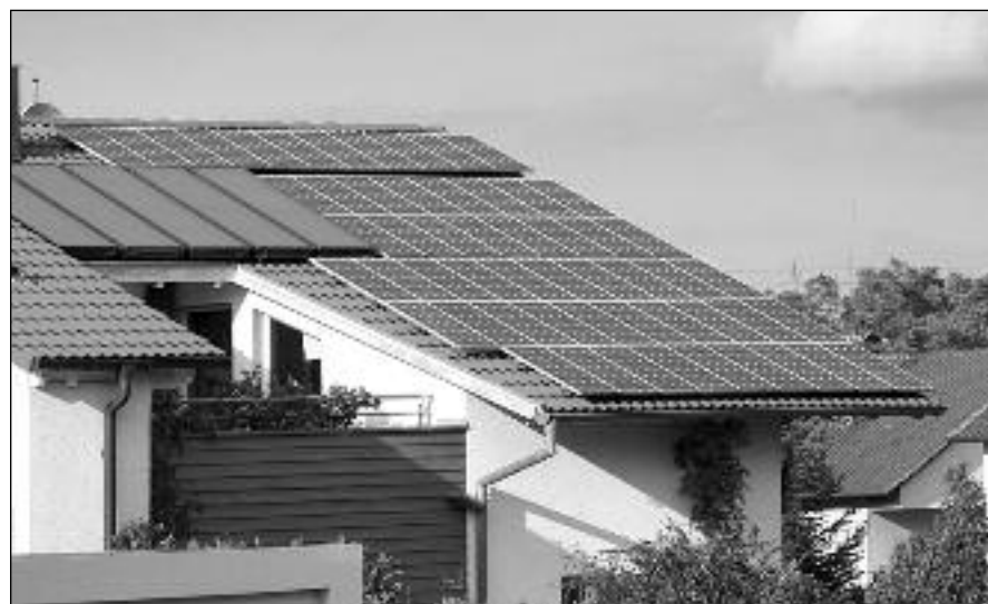
Home Solar System.
