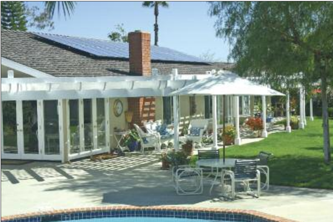
This 5.2 kW system recently installed in San Juan Capistrano covers 100% of the household electrical usage.
